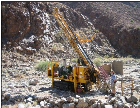
Photograph 7: This photograph shows one of the larger drill-rigs used by Teck to drill the deeper drillholes at the Haib eastern anomaly area. This rig is situated in the Volstruisrivier at Haib.
