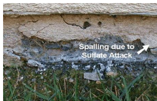
Figure 1. Example case of sulfate attack on concrete
