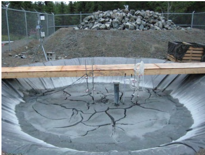
Figure 20.3: In-Situ Cells – Tailings cell in foreground, waste rock (serpentinized dunite) in background diameter of tailings cells is 5 m
