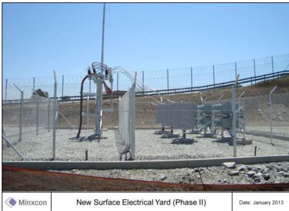
Figure 54: New Surface Electric Yard for Phase II
