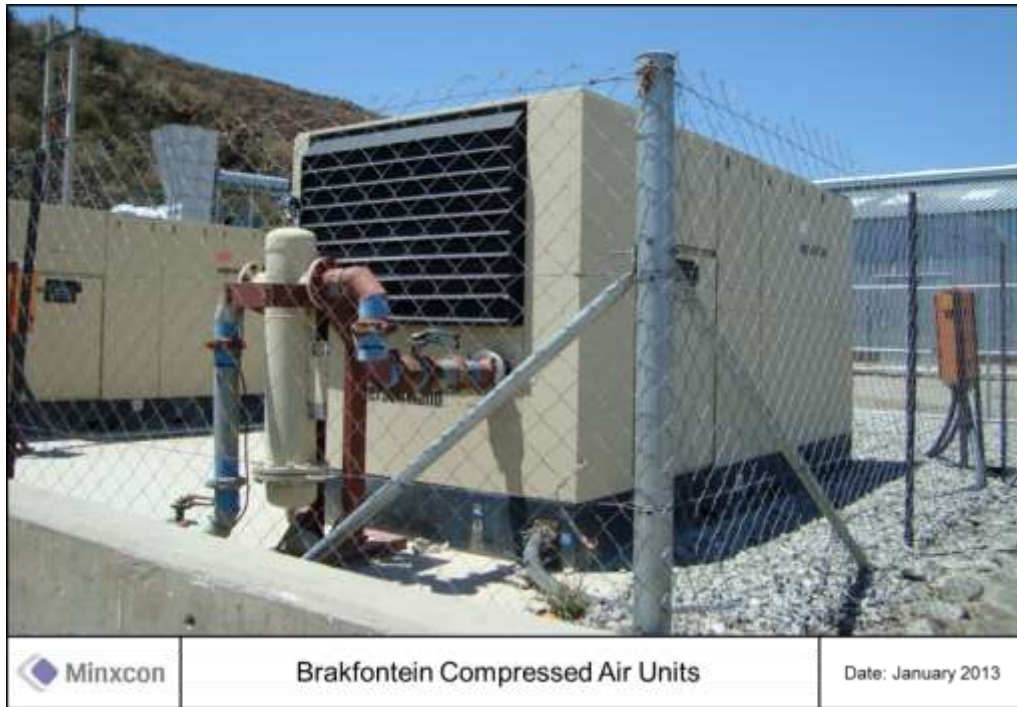
Figure 59: Compressed Air Units at Brakfontein
