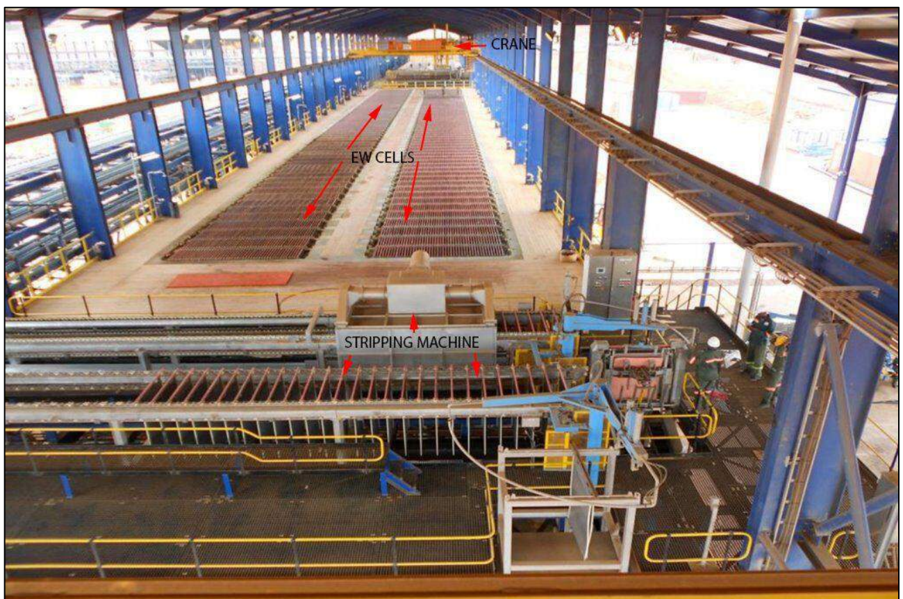
Figure 17-16 Internal View of Electrowinning Plant
